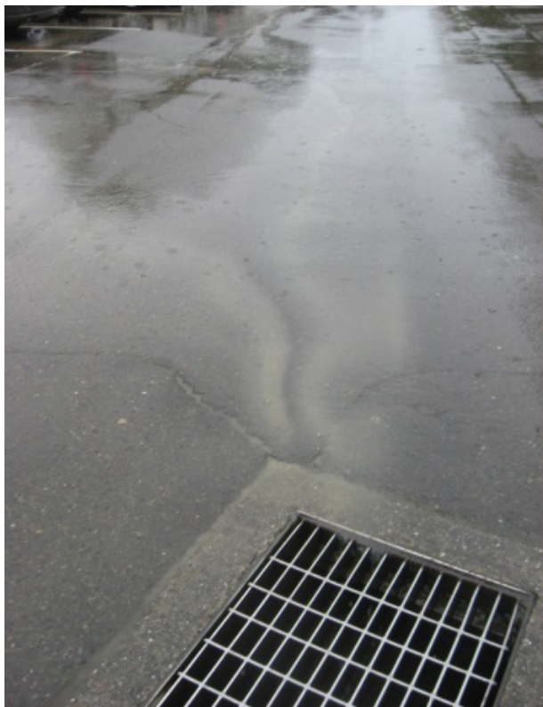
Drain Inlet - Campus
